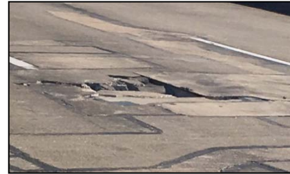
Hole Through Bridge
