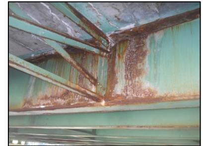
Bridge Girder Corrosion
